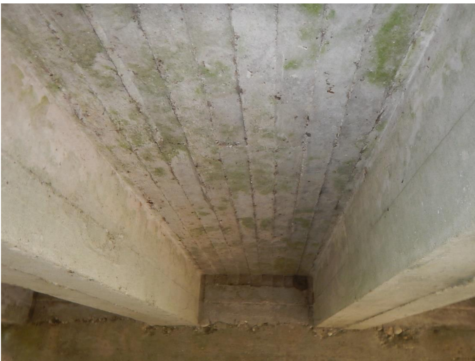
Plate 10: Underside view of bridge- north girder end. Note the "T" joints and 2x4 marks visible under the deck.
