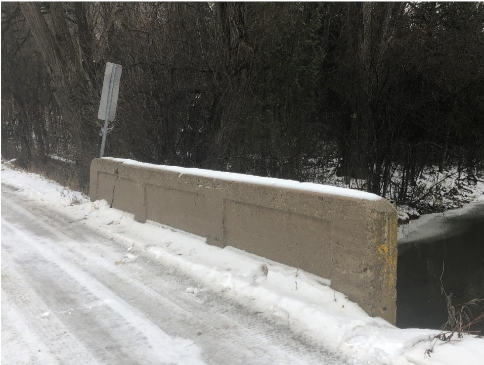
Plate 4: View of the east parapet barrier.
