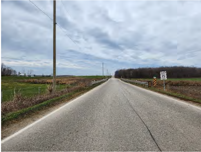
Figure 17: Northern approach to subject bridge and view of object marker signs and steel guardrails, looking south (A.S.I., 2022).
