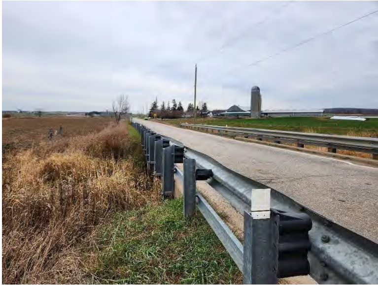
Figure 15: Detail view of modified side mount steel beam guide rail, which replaced the original concrete barriers in 2010, looking northeast. (A.S.I., 2022).
