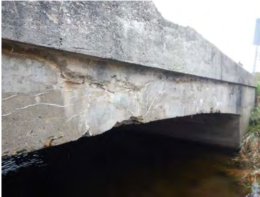
North face showing severe scaling, spalling and cracking with efflorescent staining
