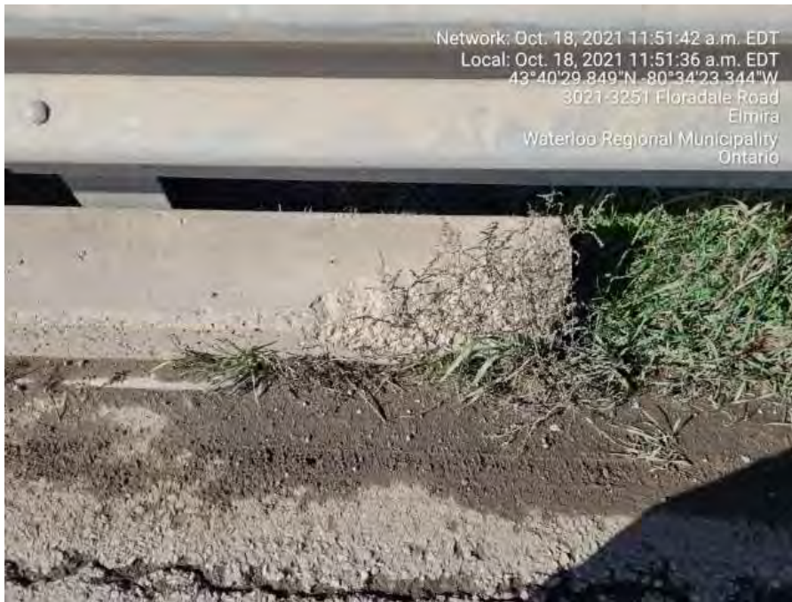
Northwest curb showing severe spalling
