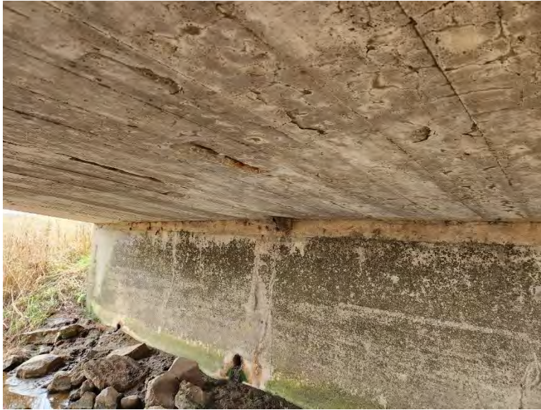
Figure 13: Detail view of north abutment showing cracks in concrete on underside, looking northwest (A.S.I., 2022).
