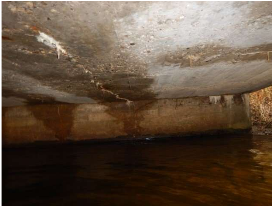
Soffit looking east showing narrow cracks with efflorescence staining and stalactite formation
