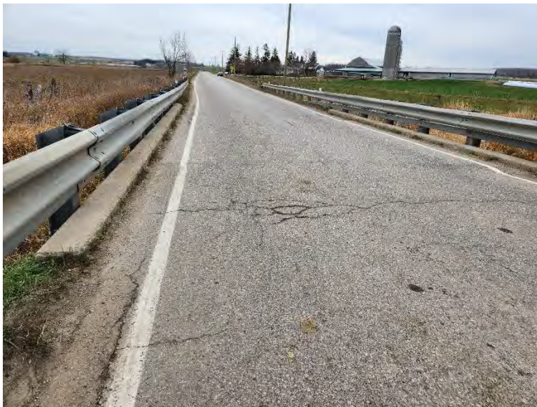
Figure 16: Detail view of bridge deck showing concrete curbs and cracks in the asphalt, looking northeast (A.S.I., 2022).
