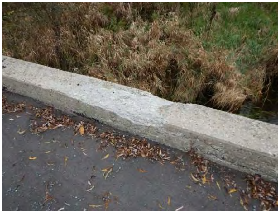
North curb showing severe scaling and spalling
