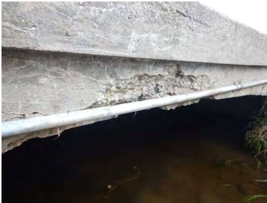
South soffit exterior showing severe spalling with exposed and corroded reinforcing steel
