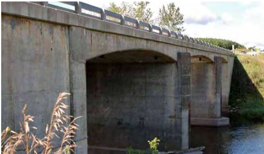
Figure 20: Grand River Bridge carrying Highway 109 over the Grand River (Benjamin et al., 2013).
