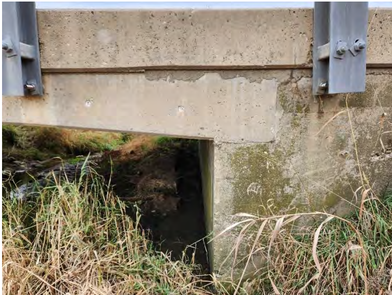
Figure 14: Detail view of the concrete abutment and wingwall connection on the southwest quadrant, looking east (A.S.I., 2022).
