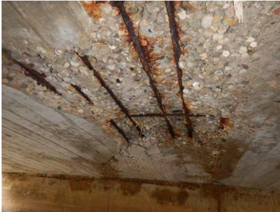
Soffit looking west showing severe spalling with exposed and corroded reinforcing steel
