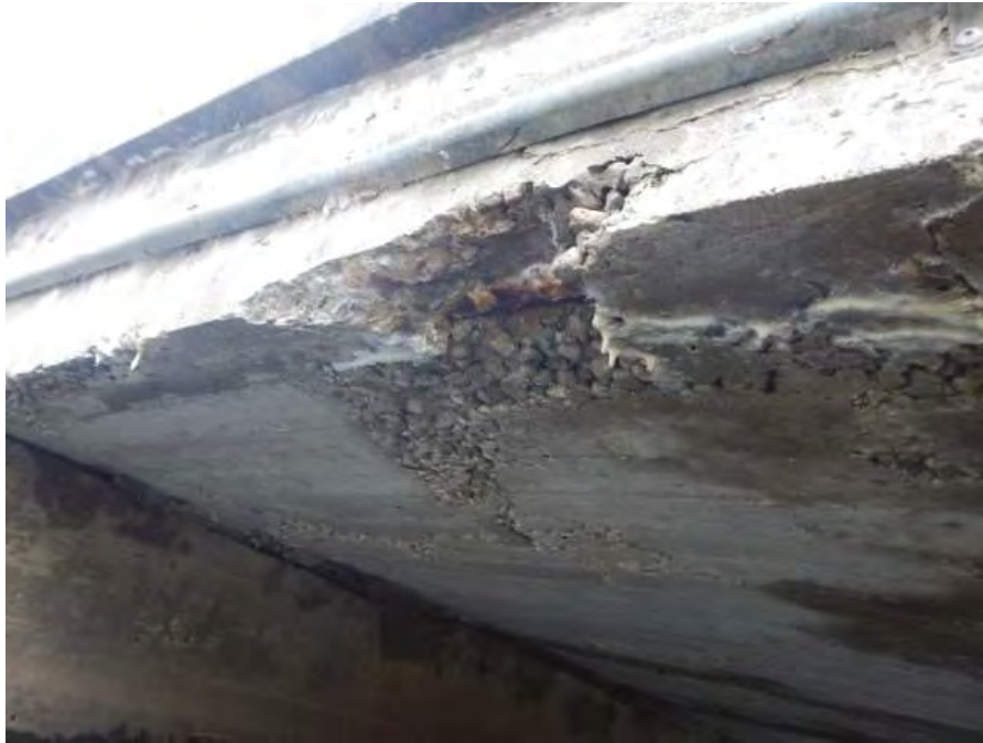
South soffit exterior showing severe spalling with exposed and corroded reinforcing steel
