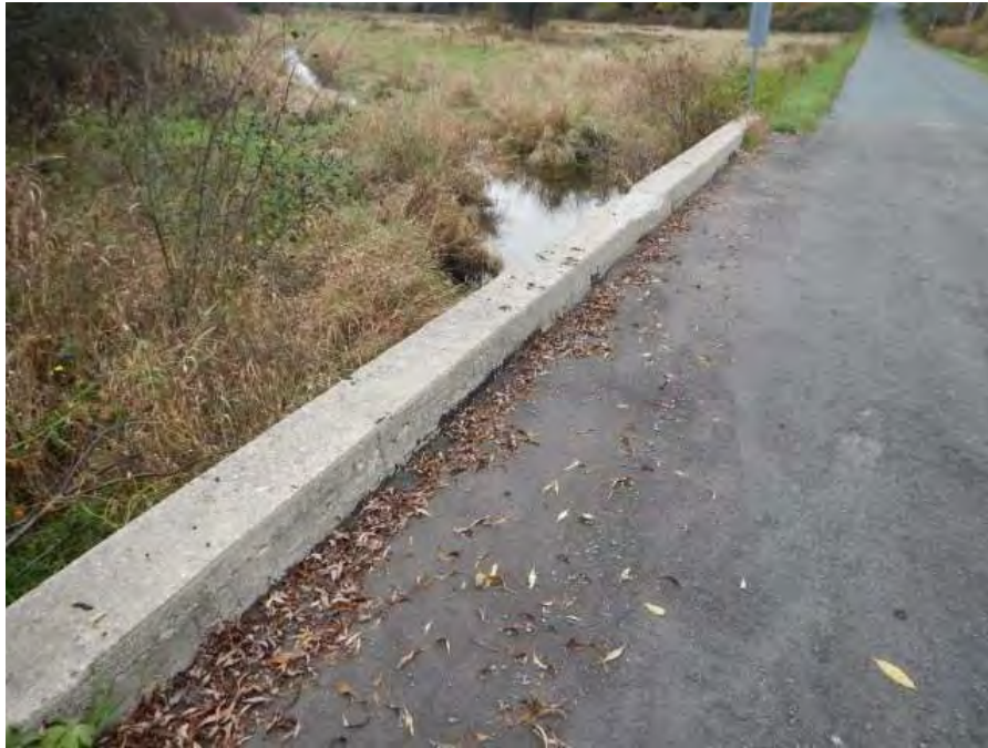
South curb showing severe scaling and spalling
