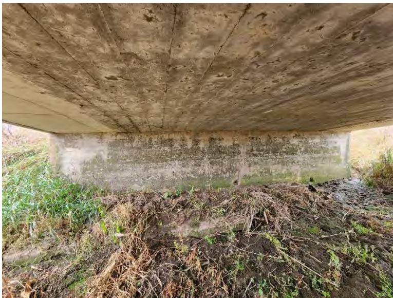
Figure 12: Detail view of soffit and north face of south abutment, looking south. Note the board formwork casting marks on the soffit (A.S.I., 2022).
