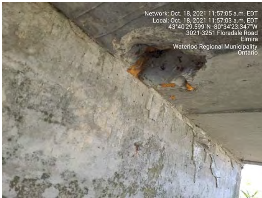
Soffit looking east showing severe spalling
